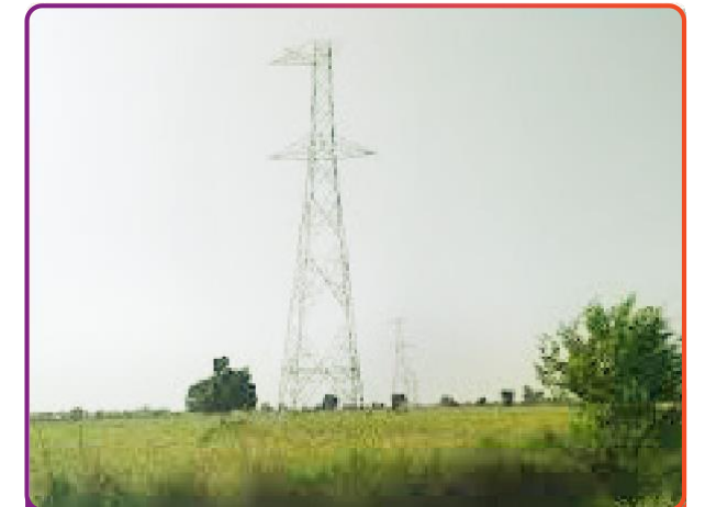
765kV Ghatampur TPS-Agra SC line
